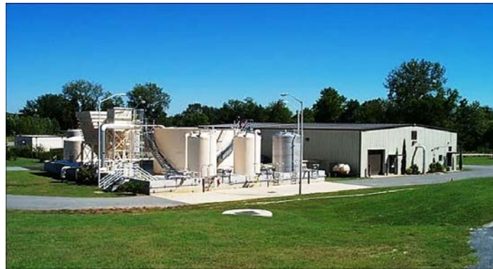
Figure 3: Pump and Treat Water Treatment System
