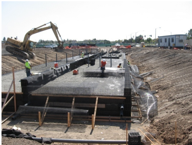
Figure 10: Photograph of Below-Ground Gravel Media Bioreactor Chambers
