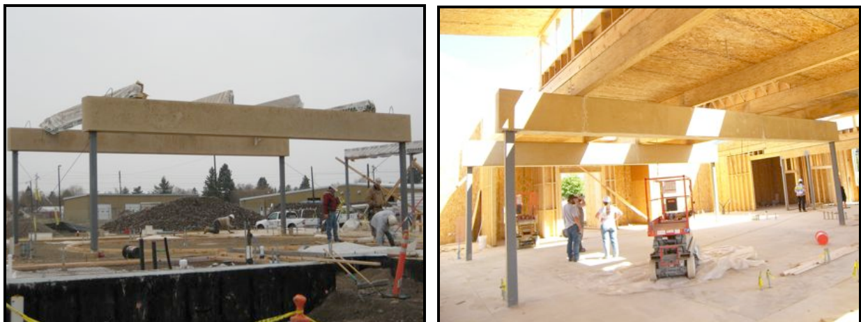
Figure 1: Load Bearing Beams at Various Stages During Construction (Missoula Federal Credit Union)
