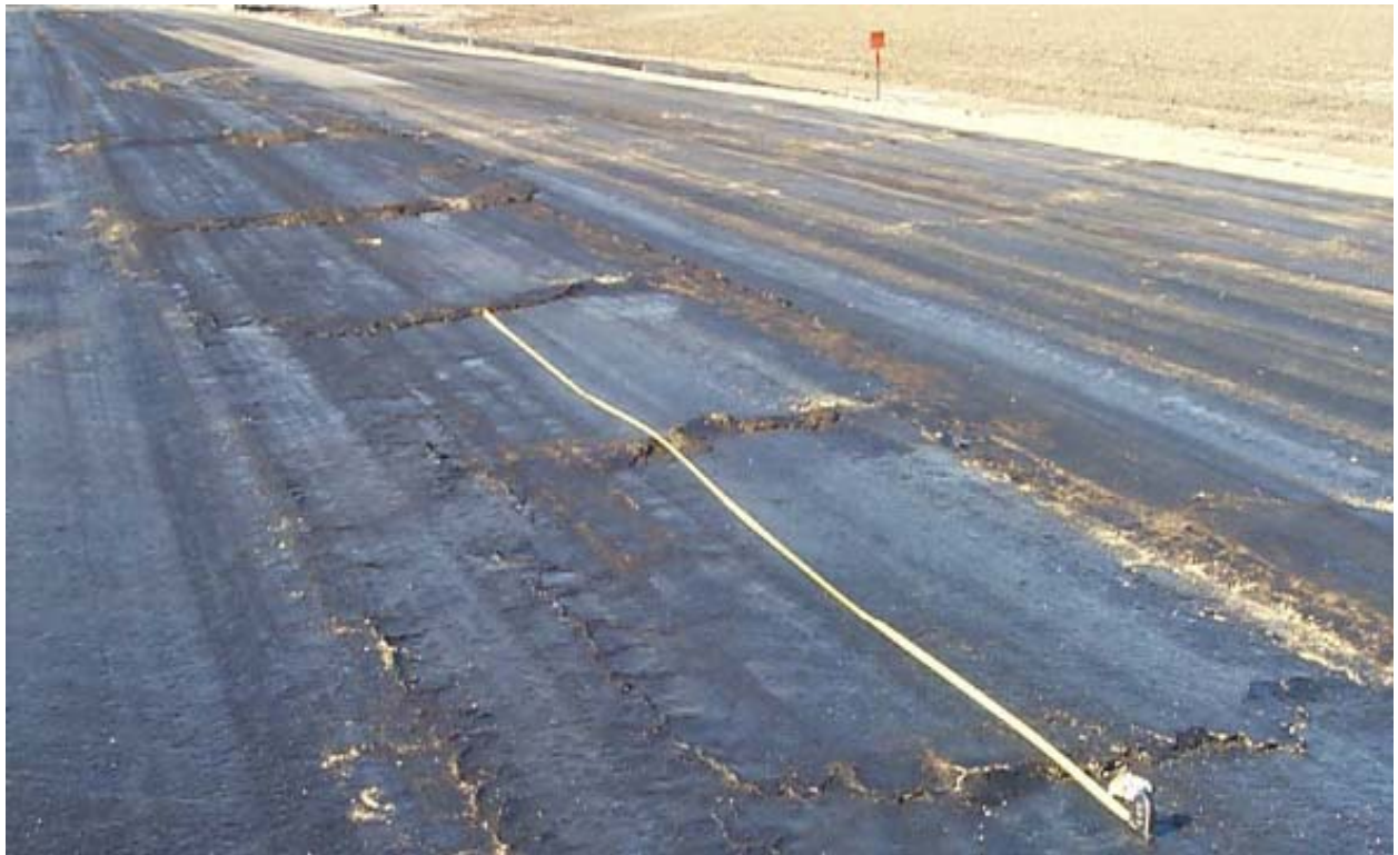
Figure 3. Typical damage to a highway pavement due to ettringite-induced swelling 12
