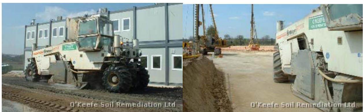
Figure 2. Overview of lime stabilisation technology: mixing hydraulic binder to soft soil and compacting it for a durable hard finish (courtesy of The Concrete Centre, UK)
