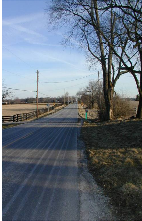
Fig.1 Failing Delaware County Pavement
