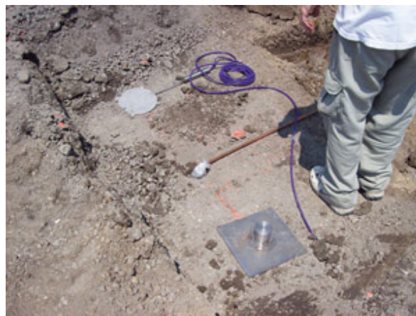
Fig. 7 OSU pavement instrumentation installed at bottom of FDR layer (left to right) — pressure cell, pore pressure device and LVDT base
