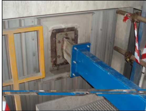
Picture 1: Bin Venting Connection to the Combustion Chamber
