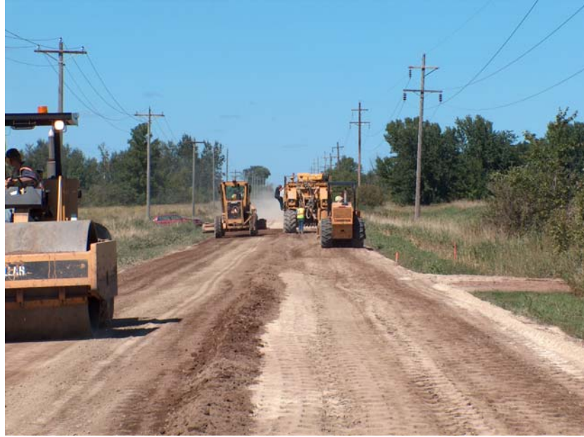
Fig. 1. Gravel surfaced County Road 53 being stabilized in situ with fly to form a firm base to for asphalt pavement
