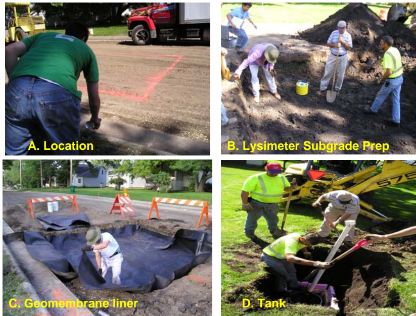
Fig. 6. Construction of pan lysimeter under 7 th Avenue before fly ash stabilized base is constructed and the street is paved. Lysimeter collects percolating water through the pavement and fly ash stabilized base for quantity and quality determination.
